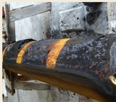
Coating scraped to measure char
